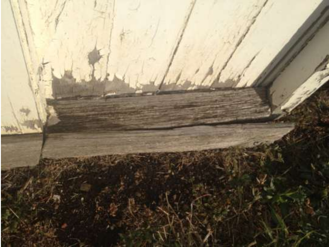
This hardwood element looks like a previous repair and it is severely deteriorated.
